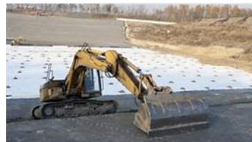
Geotextiles are used to prepare the ground before new roads are laid
